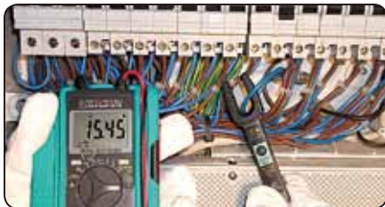
Measuring current in a Switchboard
